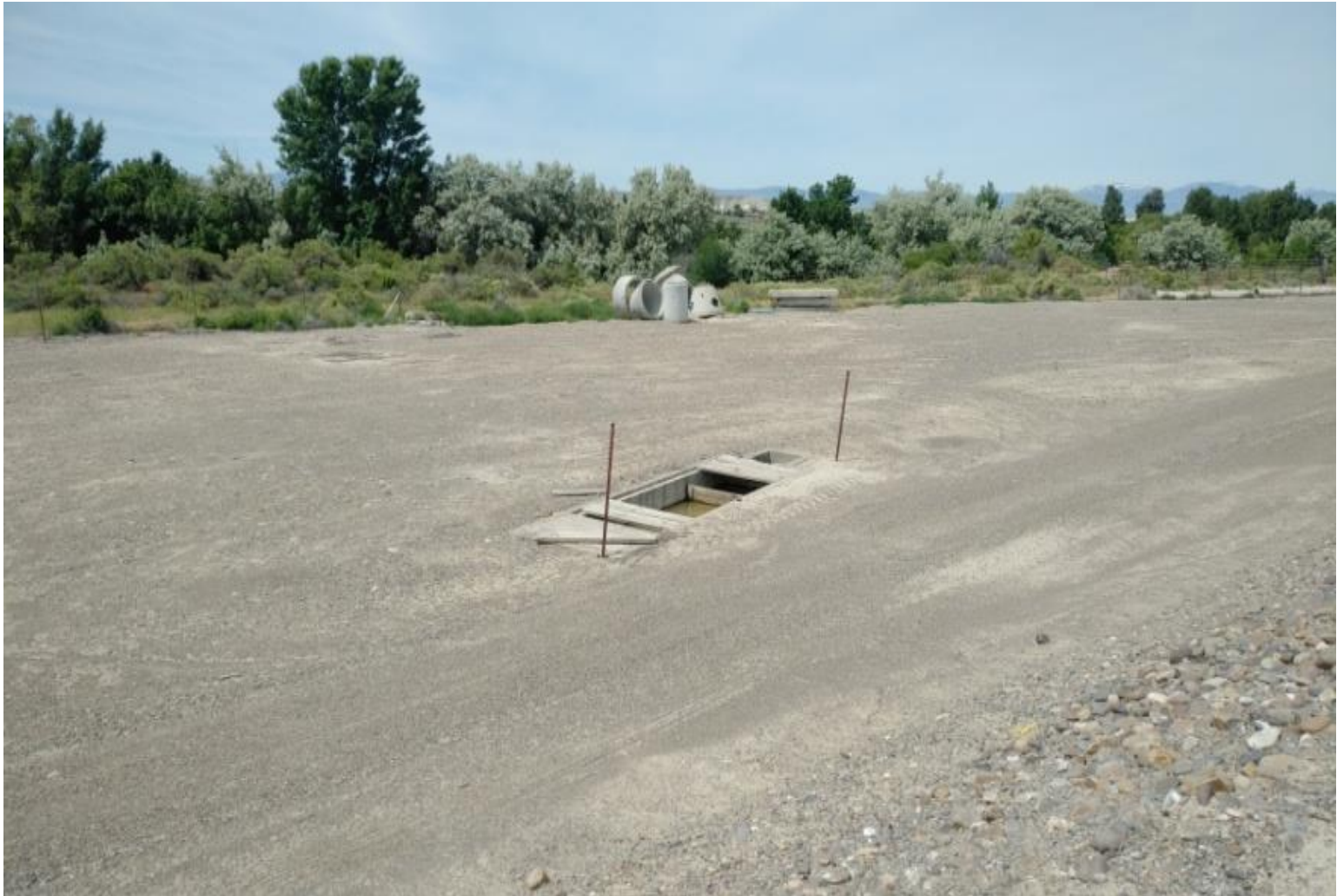
The abandoned chlorination mixing chamber showing decaying planks and some standing water (foreground: Snake River shoreline)
